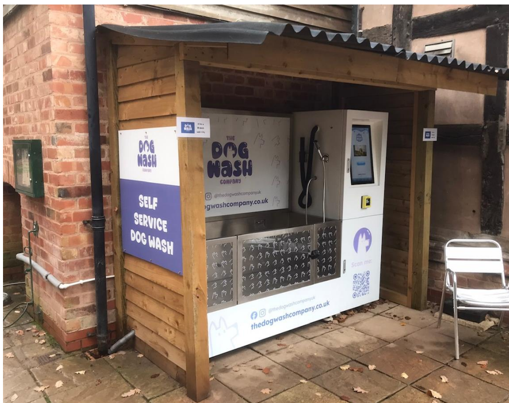
Figure 4. A Dog wash facility installed in a country park, with waste water emitting to the sewer at the bottom left of the photo.
